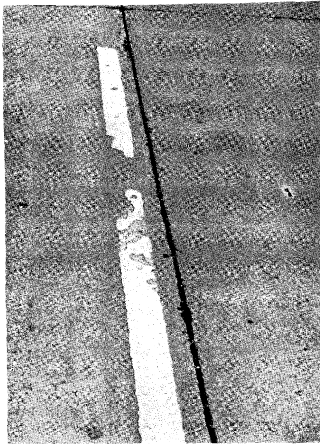
Figure 10. Poor Adhesion of Thermoplastic Material to Improperly Cleaned Surface
